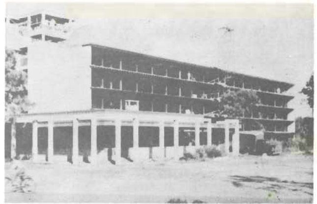
SOUTH SIDE PRESBYTERIAN HOME Bradenton, Fla. Architect—Edward Dean Wyke Builder—C. A. Friedland, Inc. Tampa, Fla.
